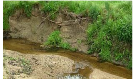
Erosion due to poor riparian buffers
